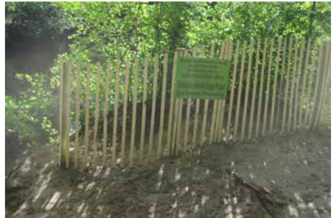
As part of a NRWA/Merrimack River Watershed Council project funded by the US Forest Service, "Expanding Riparian Buffers," and with the help of a local Eagle Scout, the eroding banks at Bertozzi Conservation Area in Groton, MA were restored with plantings of native shrubs and grasses. Photo: Al Futterman.
