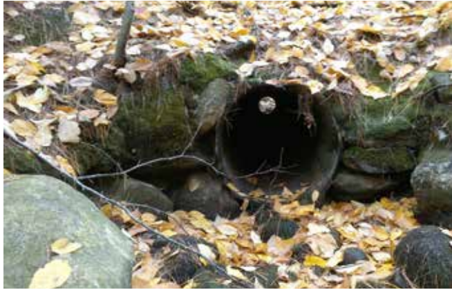
Poorly or undersized culverts can create high water velocity, turbulence, and/or inadequate water depths within the culvert leading to migration barriers for fish and other aquatic species. They also restrict natural stream flows, particularly during floods.
