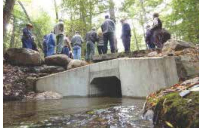
Replacing old pipe culverts with new bottomless, three-sided culverts helps provide passage for fish and other aquatic species. Such projects often necessitate the efforts of multiple partners to accomplish, such as here with Trout Unlimited's involvement with a Gulf Brook culvert in Pepperell, MA. Photo: NRWA Archives.
