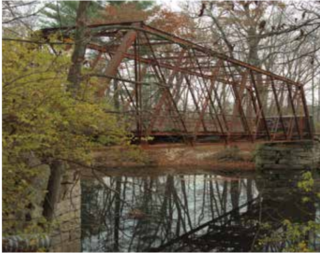
Historic Fitch's Bridge in Groton, MA, originally built in 1898, is shown here prior to being demolished in 2013 and replaced with a pedestrian-only bridge. Photo: Olin Lathrop.
